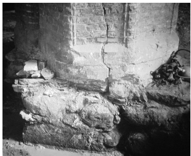
Fig. 6 Cracked pillar pedestal in the eastern part of the church (1995).
