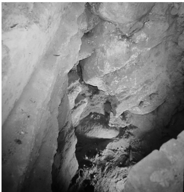
Fig. 7 Cracked stone foundation of a single pillar
